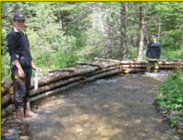
ABOVE Cheticamp River Salmon Association project biologist Julie Malouin and crew member Nicholas Aucoin at a crib structure installed to establish a bank and focus the channel in Aucoin’s Brook.
