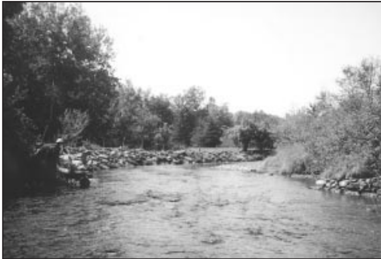
River Philip Restoration—Cumberland Co. River Enhancement Association completed 500 feet of bank stabilization (left) and installed 10 wing deflectors (picture on right is one)
